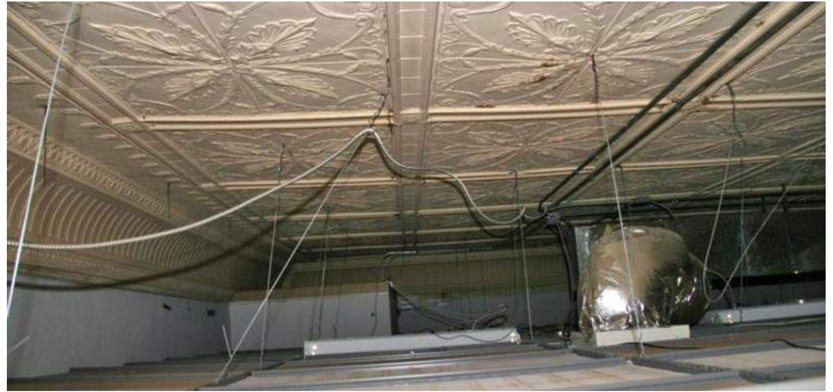
Extant tin ceiling above acoustic ceiling tiles in the 2nd floor courtroom. August 17, 2017. Spencer, Brenda ( http://khri.kansasgis.org/index.cfm?in=149-5770-0002 )
