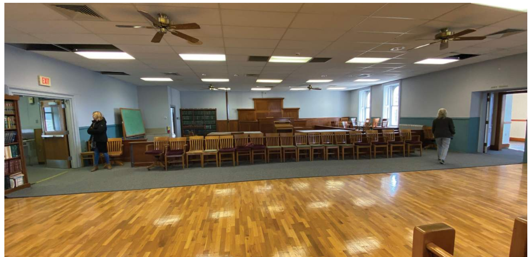
Fans and supply diffusers from modern HVAC systems cover up the historic features in the 2nd floor courtroom.
