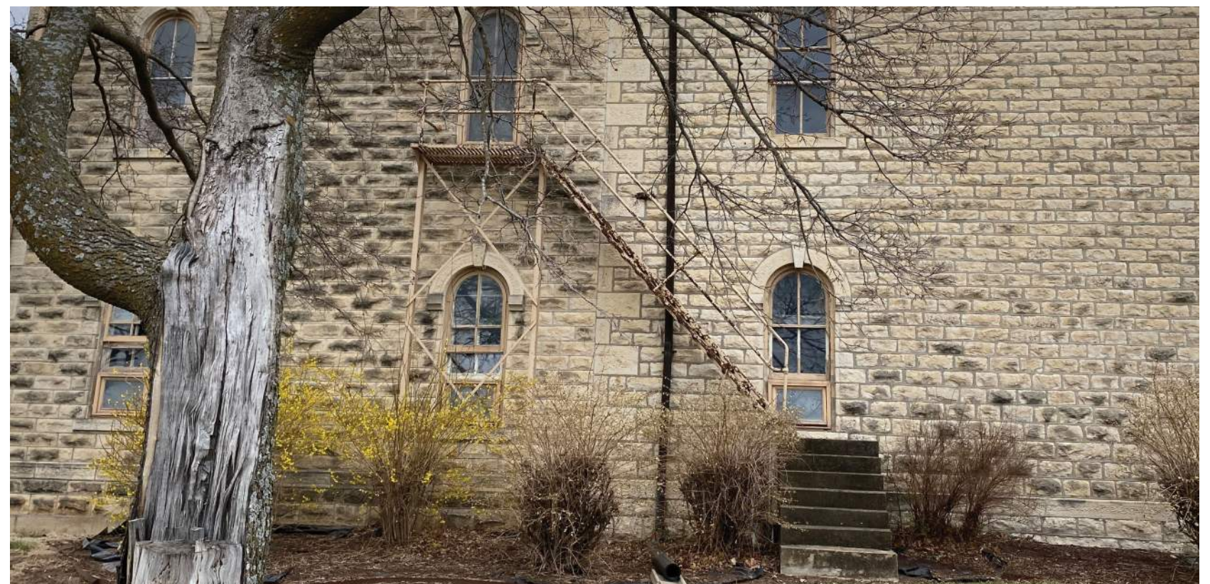
View of an existing deteriorating fire escape, accessed out of a second floor window.
